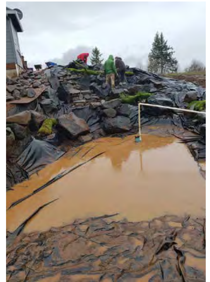
Our Team places rock in the waterfalls while evacuating rainwater from the pond area.
